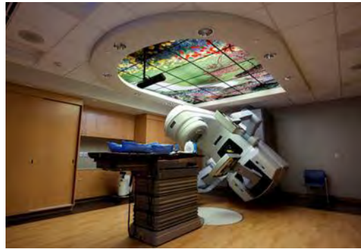
63- Clarkston Cancer Center Linac Room 12' x 10' Ceiling Backlit-Installation
